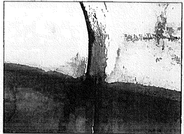
Spalling with exposed rebar and opening at joint.
